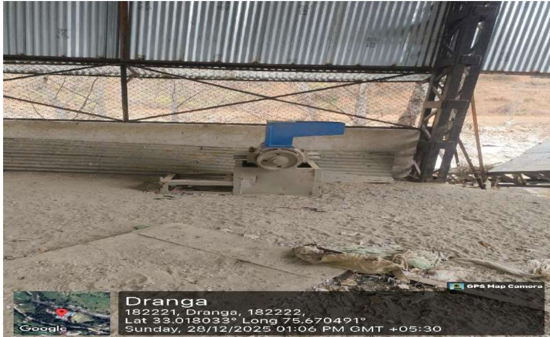
Municipal Committee Bhaderwah- MRF shed partially damaged
