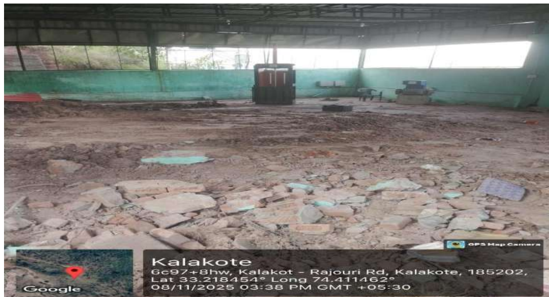
Municipal Committee Kalakote – MRF shed partially damaged.
